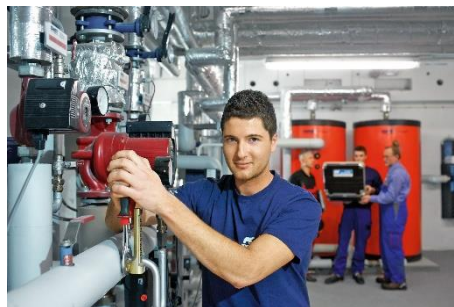
Dussmann Technical Solutions: Cooling and air conditioning technology
